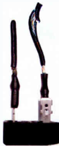
Figure 3: High current combined with insufficient ventilation and nonsolder crimp connections added up to crispy wiring.
