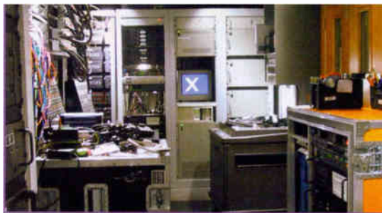
Hit Factory/Criteria machine room
