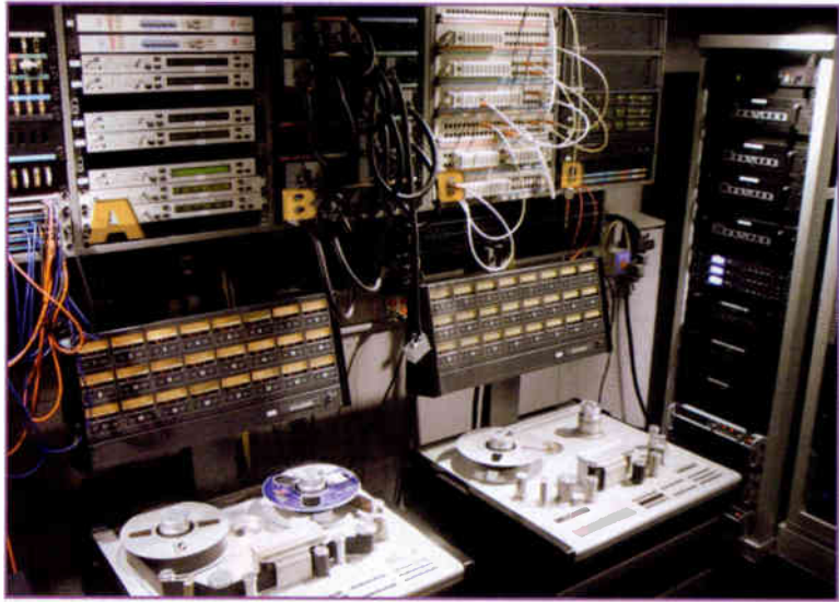
Patch panels keep audio, analog video, data and digital audio cables organized.
