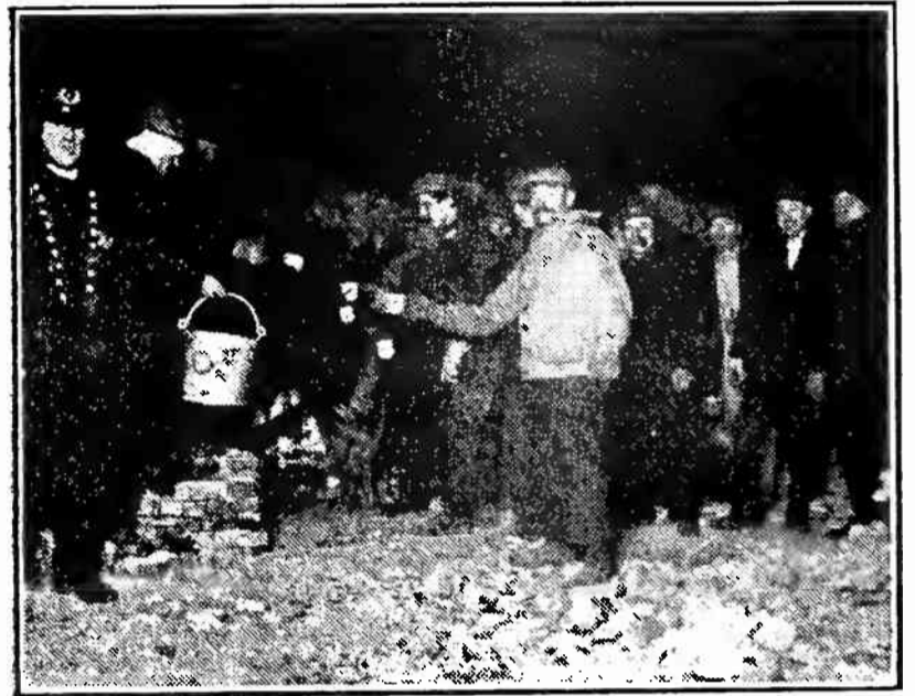
THE NIGHT SHIFT GETTING SOME COFFEE Ever since the fire there has been about 2,000 men working night and day clearing away wreckage and doing reconstruction work.
