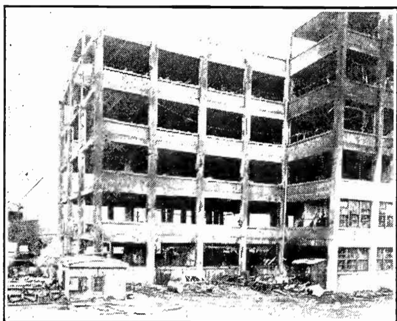
This is what happened when a fire hose was turned on the red hot columns on third floor of the Record Plant.
