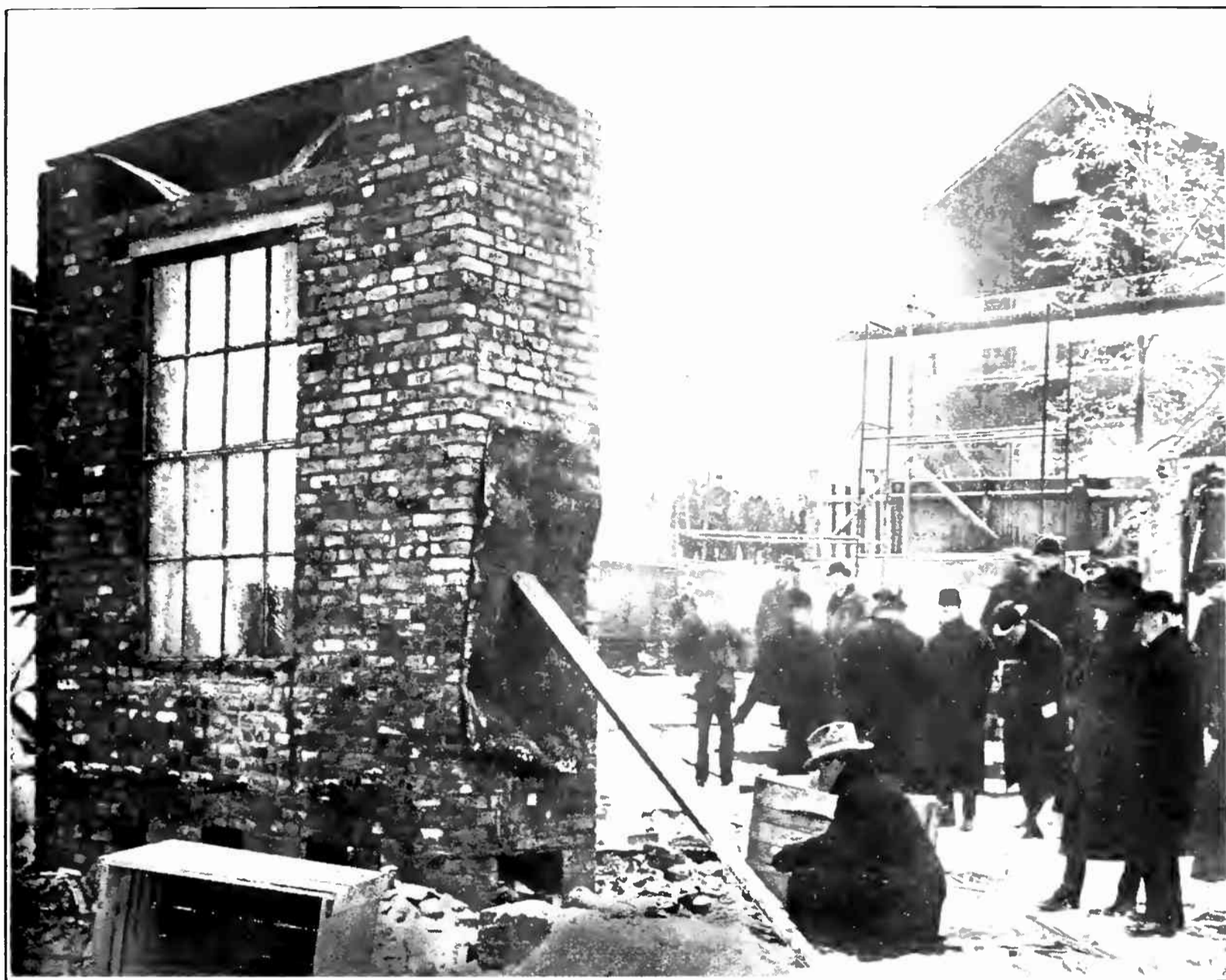
SPECIALLY CONSTRUCTED CHIMNEY FOR TESTING TWO KINDS OF WIRE-GLASS WINDOWS WITH STEEL FRAMES AND SASH
