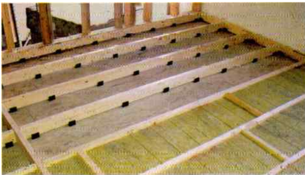
Fig. 1: Floating floor construction. Note how the spacers ("U-Boats" by Auralex) are placed to isolate the floor support boards from the "real" floor. (Photo by Jeff D. Szymanski)
