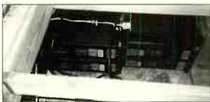
Three IT-1220's paired with three AR-1220 Voltage Regulators visible under the floor at Vital Recording.
