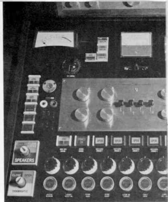
The reverse side of the entertainment center is easily accessible in the event some circuitry troubles occur (wood doors normally hide the elaborate circuit wiring and components revealed here). The control panel above gives Mr. Genin fingertip control over all functions of his system.
