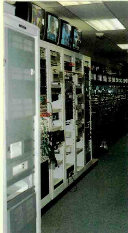
Above: The machine room.
