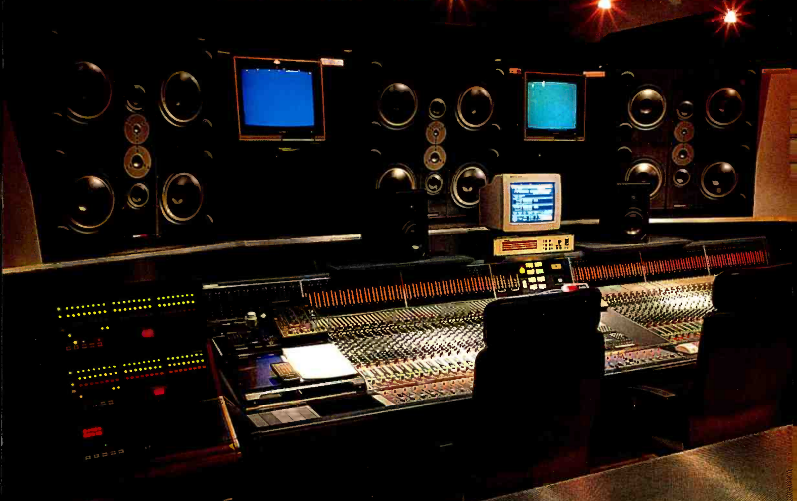
LCR DynaudioAcoustics M4 monitors and Neve VR72 console dominate the Pierce control room
