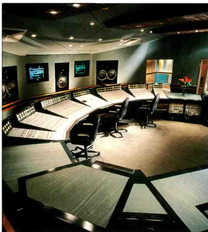
Codenamed 'Bluestone', the highly customised SSL 96-input mixing console recently installed at The Hit Factory Digital Studios in New York. Discrete Systems Technical Director David Bell specified the console's 'in-the-round' appearance to provide the engineer 'with substantial amounts of readily accessible table top workspace'—a keynote that Bell believes to have been overlooked by other solutions
