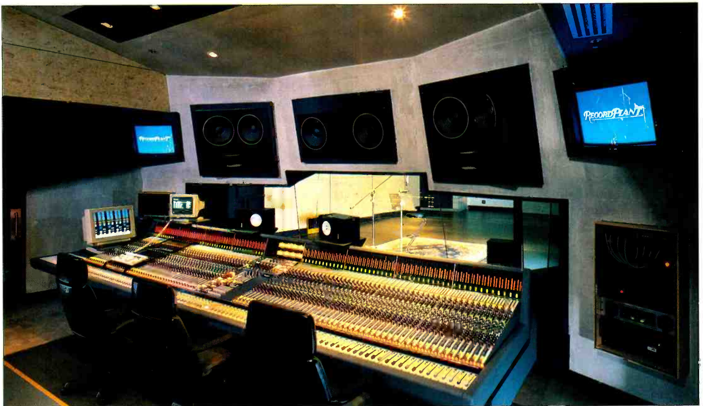
View of NEVE 1, which houses a 96-input Neve VRSP Legend console with GML Moving Fader automation and recall. Each of the two new studio suites functions as a self-contained environment with private lounge, bathroom and kitchen, as well as control room and recording areas
