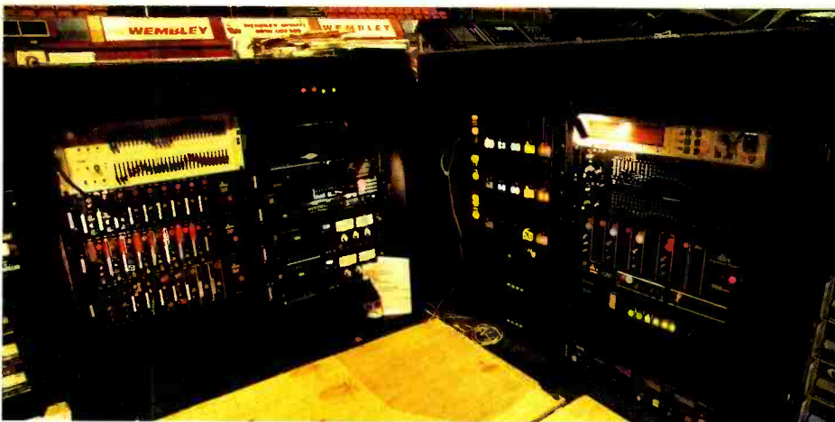
Prism digital control racks and drive rack
