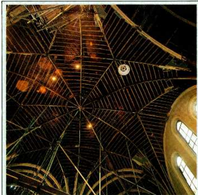
The ceiling of the large missionary hall in Lyndhurst Hall, Hampstead, the new home for Air Studios, London, has now been completely stripped back leaving this unusual star-shaped timber pattern. Full story of the studios' progress can be found on page 55 of this issue.
