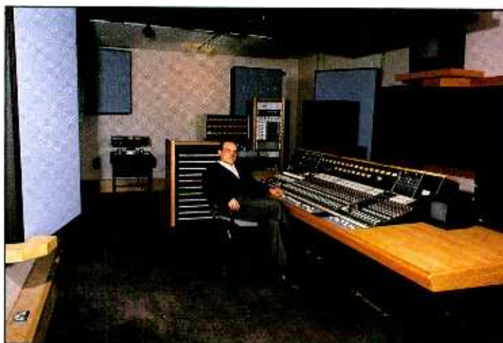
Recording Architecture Black Box acoustic panels installed at CTS Studios
