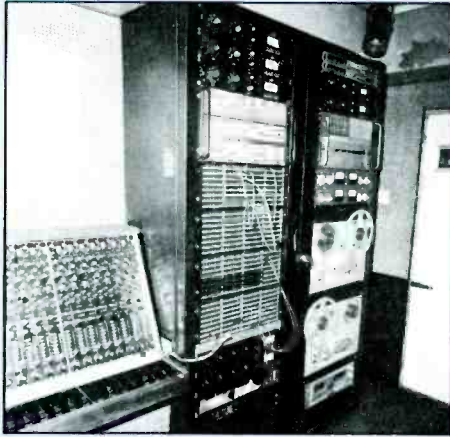
Equipment racks rear truck
