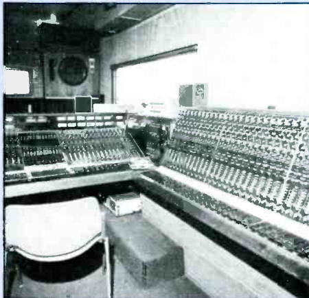
Pumacrest mixing facilities
