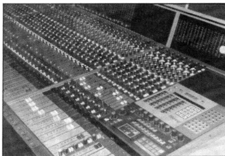
Neve 8108 console with touch sensitive routing and monitoring in foreground.
