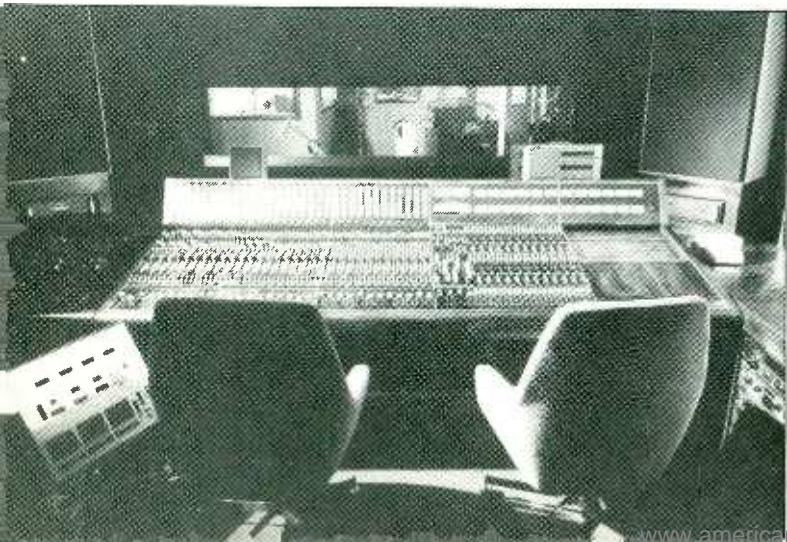
Below: Trident TSM desk installed at Good Earth Studio
