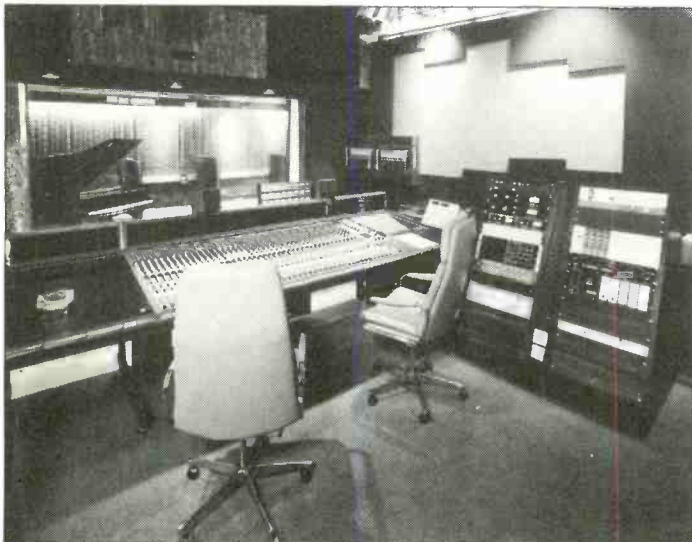
Marquee's new model 542 automated console
