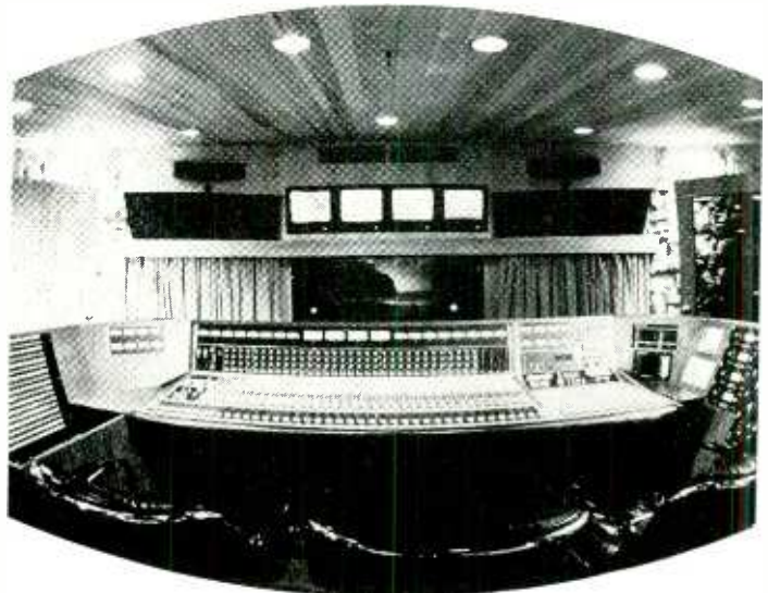
The control room at Threshold is typical of present-day multitrack recording installations
