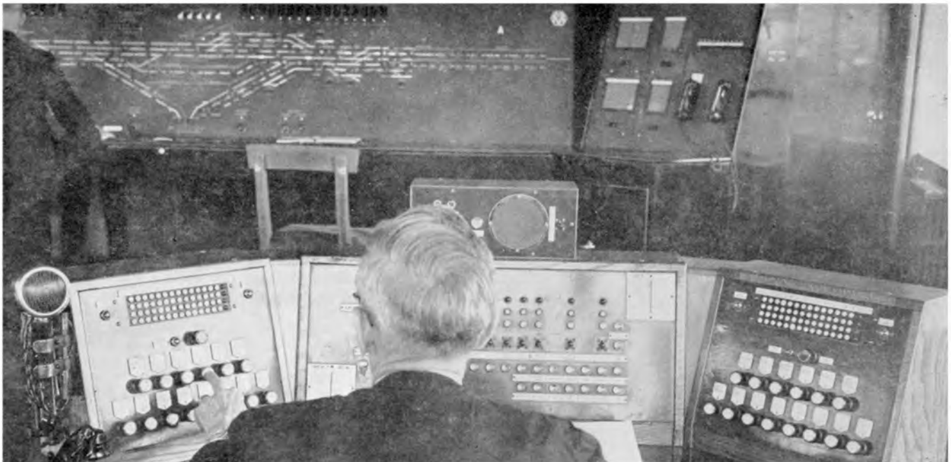
The above photograph shows the train control operator at the control panel at Stratford Station. The position of this desk in the signal box allows the operator to check with the train signalling system and so determine which announcement has to be relayed.
