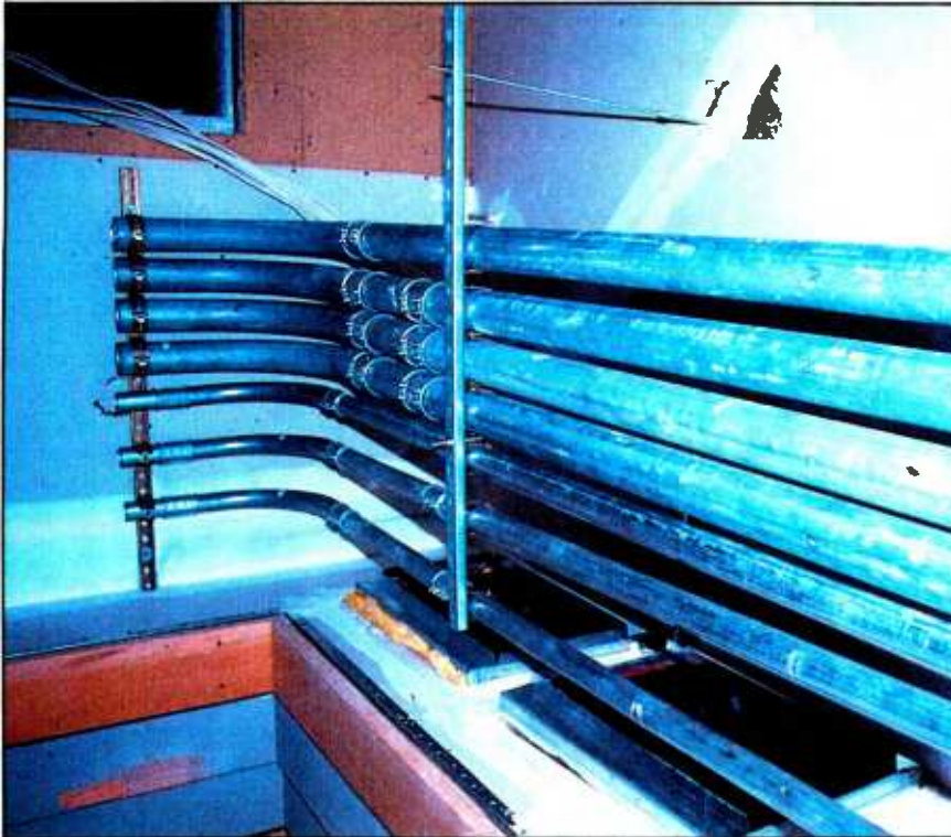
Photo 3. Multiple ceiling conduits contain audio, video, MIDI, Synclavier, telephone and spare wiring.
