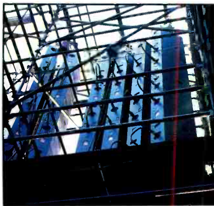
Figure 5. At Irvine Meadows Amphitheater, the Prism system was stacked vertically within the facility's scaffolding system on each side of the stage.
