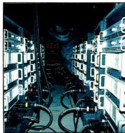
Figure 12. Crown PSA-2 and Micro tech 1200 power amplifiers are used to drive the system. Note custom power distribution panel in background.
