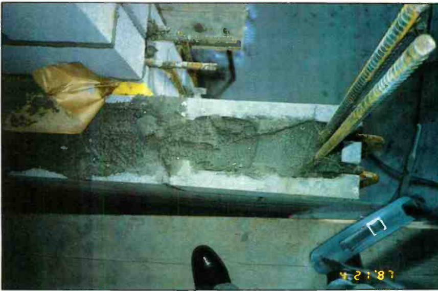
Construction at Spectrum Studios included double walls of reinforced grout filled concrete block completely decoupled from the other wall.
