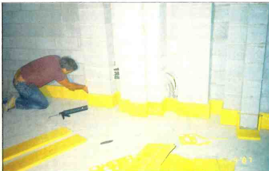
Installation of isolation material along low-frequency quadratic residue diffuser in Studio A.
