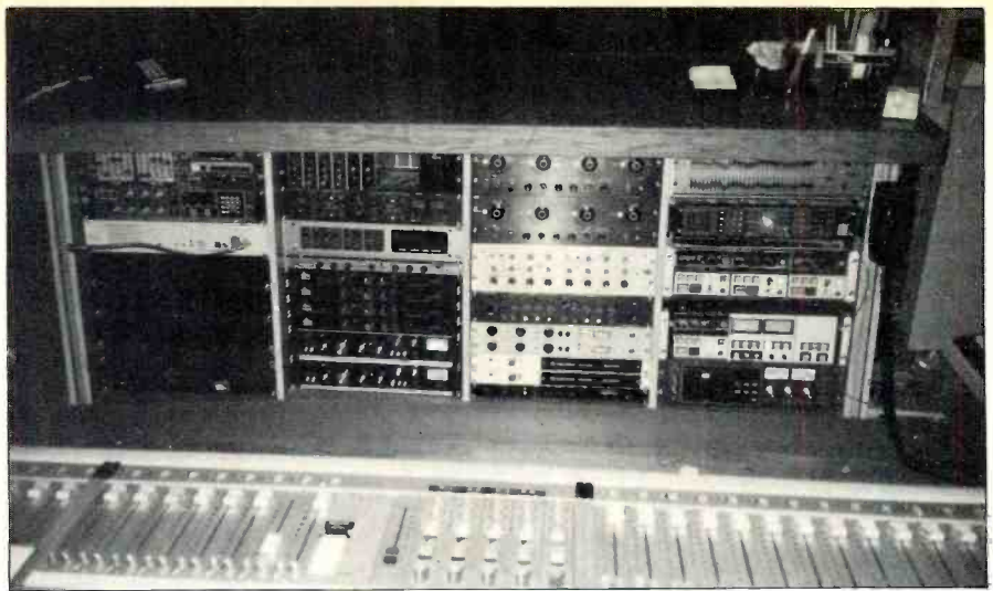
Outboard equipment in the Post Group's Studio A includes a Lexicon Super Prime Time, AMS DMX-15S delay, dbx compressor limiters, and a Quantec Room Simulator.
