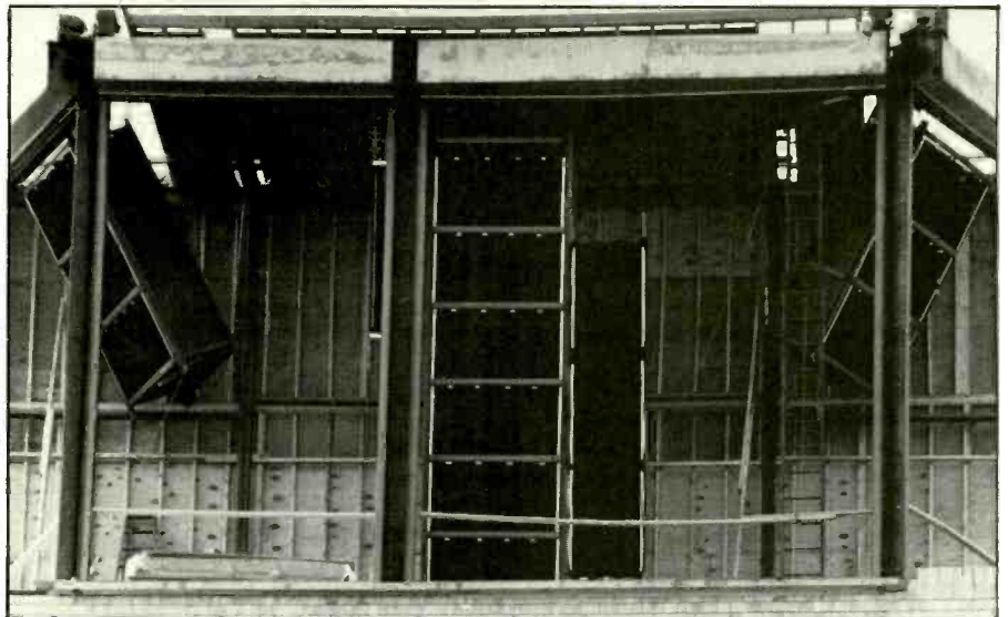
Central Speaker Cluster during construction. Shown at top of the page are low-frequency side-fill cabinets, and below the front-facing center low-frequency and mid-frequency cabinets for the stadium's North End.
