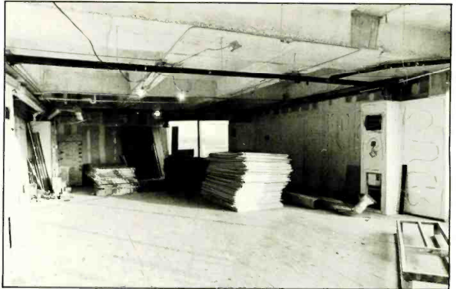
Building space stripped prior to studio construction. This view is from the future control-room area through the studio recording area and office space.
