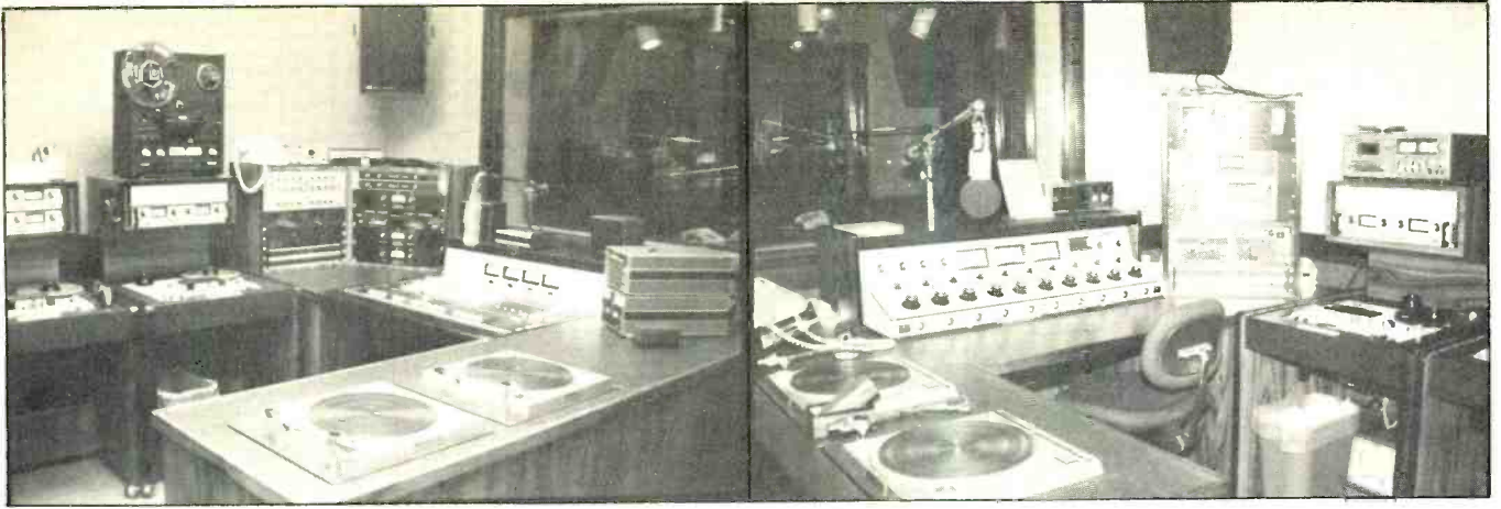
KGB-FM four-track production studio, one of a pair of multitrack rooms available for in-house commercials and PSAs.
