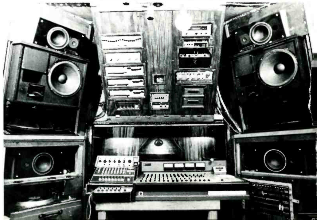
FIGURE 1: FyF control room monitoring environment. The smaller speakers at the top and bottom comprise the FyF System monitors.
