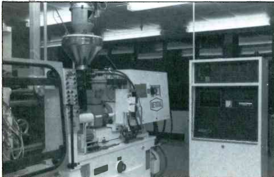
Detail of press and control panel
