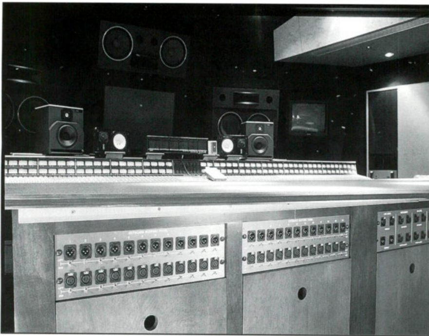
Figure 5. The back of each outboard rack is fitted with audio, video and MIDI tie-lines. This allows processors and musical equipment to be used free-standing on the table top surface.
