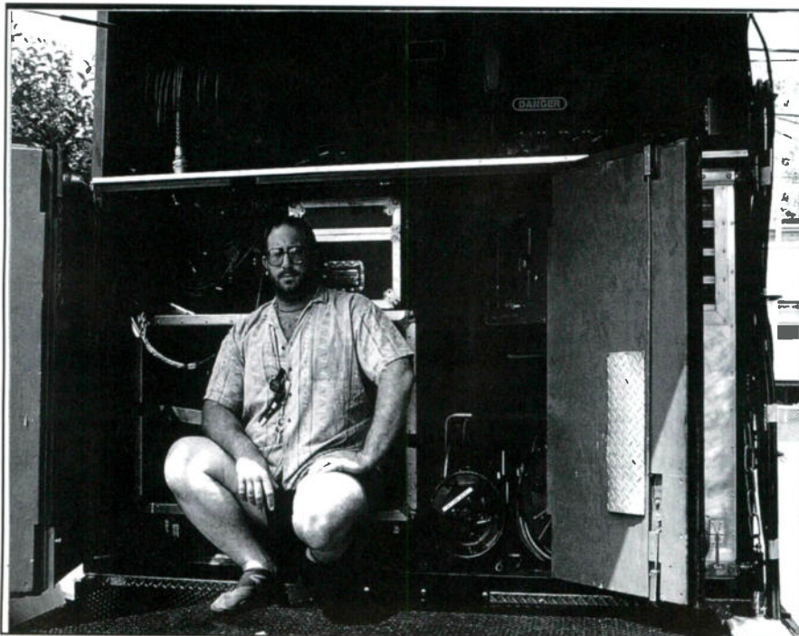
Figure 3. Steve Remote sits along side of air ducts that are within reach for future hook up for the truck's rear extension
