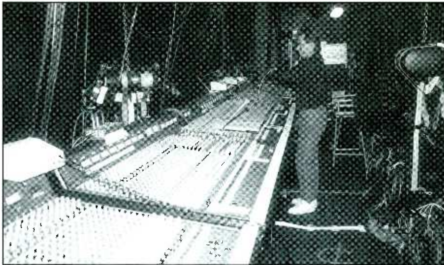
Figure 2. These four Ramsa WR-S-840 consoles handled sound reinforcement for the room and were on the specially-built platform in the theater. Burns Audio used engineer-mixer Mike Abbott who is seen during a rehearsal
