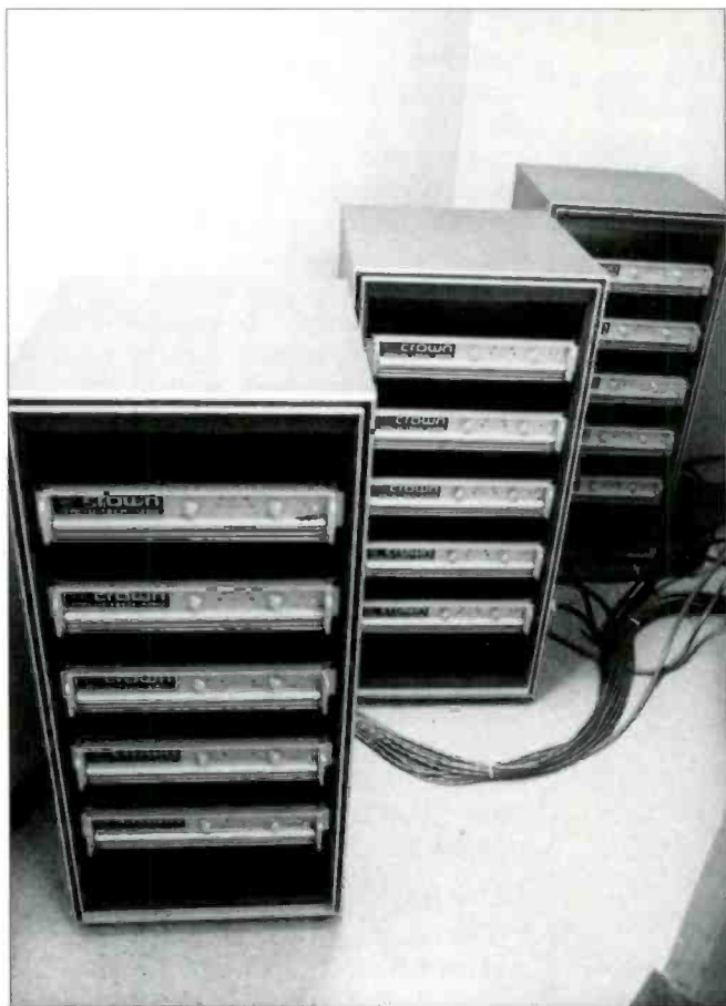
Figure 4. These racks of Crown Macro-Tech amps are one of two such located overhead, just above the house right cluster.
