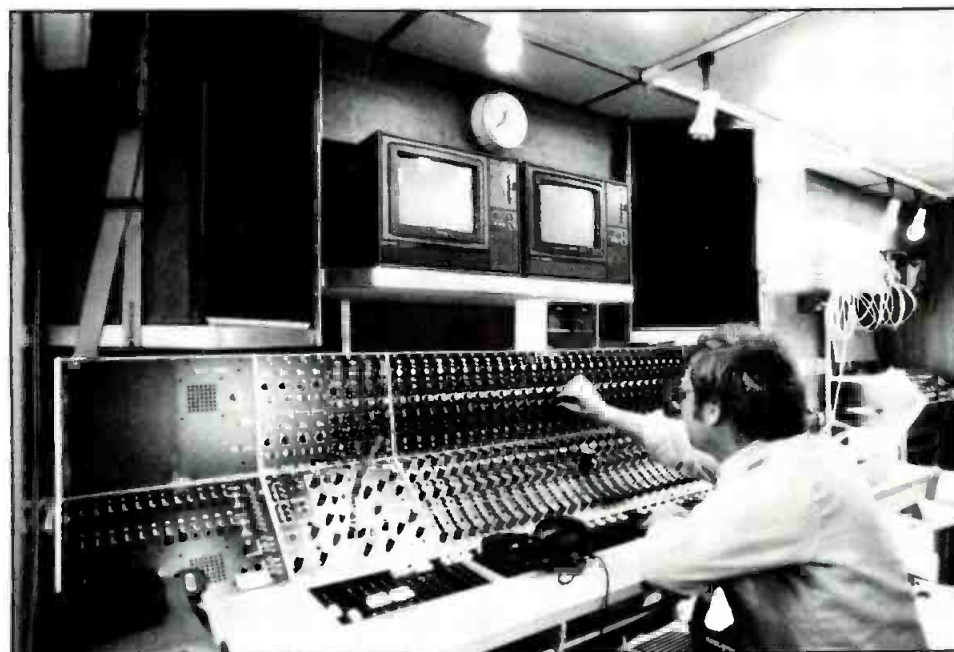
Figure 7. Control room of a mobile studio featuring a 30-channel Glen Sound mixing desk and Studer B62 recorders.
