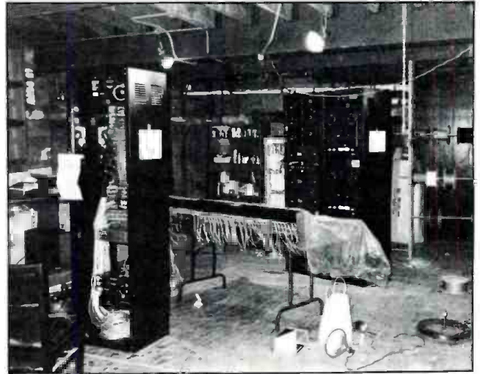
Figure 3. The Virginia Center's control room set up in the Alpha basement.
