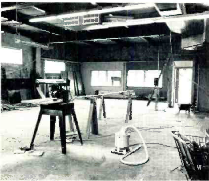
The gutted shell as seen facing the future site of the control room.
