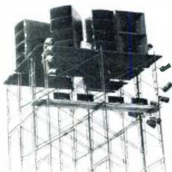
Main Tower #1 (40 x 60 horns in 2nd tier not in final position.)
