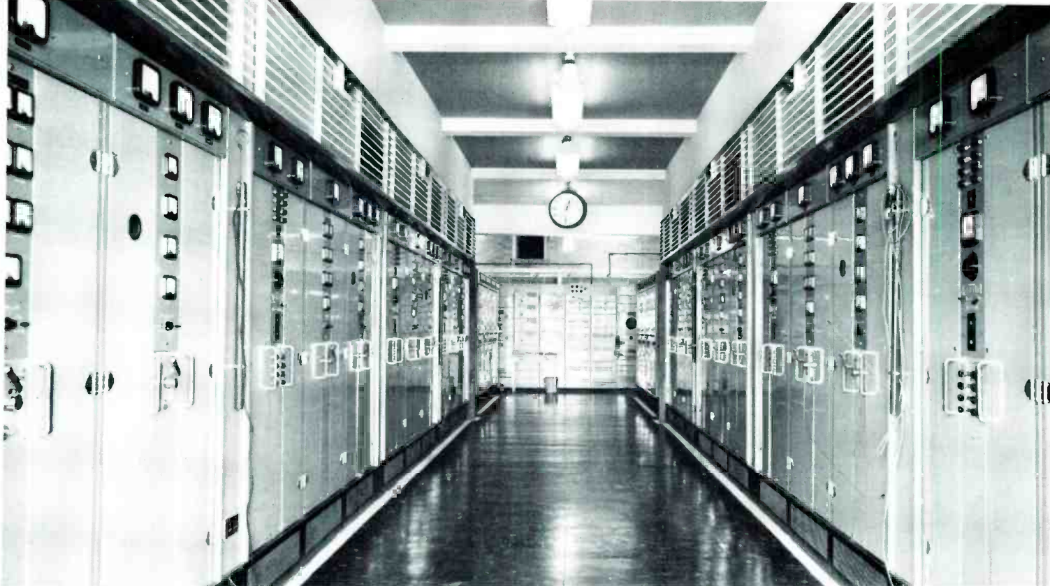
Figure 1. Medium sized BBC transmitter facility. Sandale, Northern England. BBC photo.
