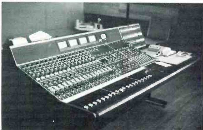
The other control room has a (more or less) stock Neve console that was installed with a great rapidity and without a hitch. It has 16 channels in, and as many out, and is currently being modified.
