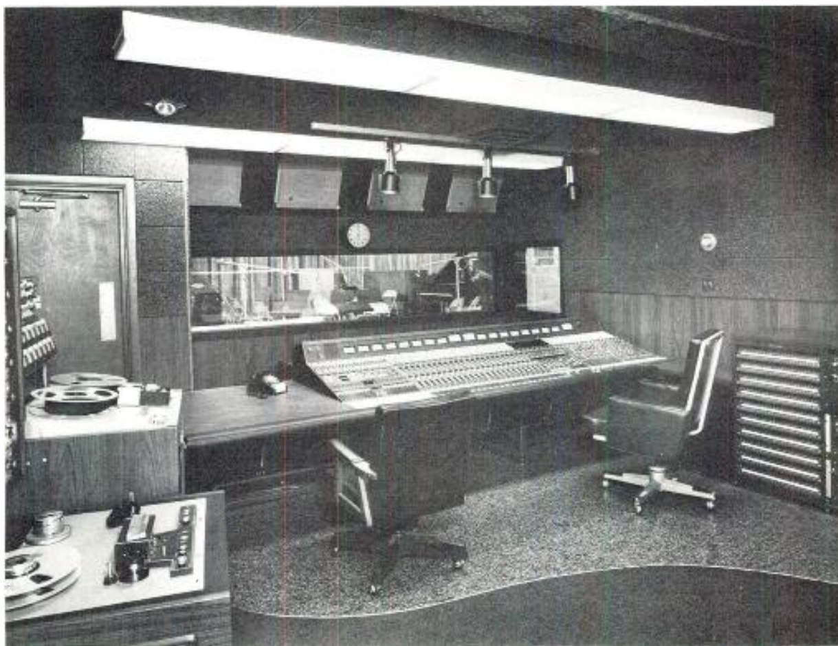
Figure 1. Studio A master control. The Neve console looks into the studio and permits all corners to be seen. At the extreme left, the sixteen track 3M and eight-track Scully are visible.
