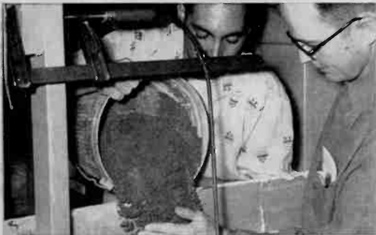
Pouring concrete into the wall cavity between the two systems was a two-man job. The concrete added mass to the wall on which the speakers were mounted, thereby reducing resonances.
