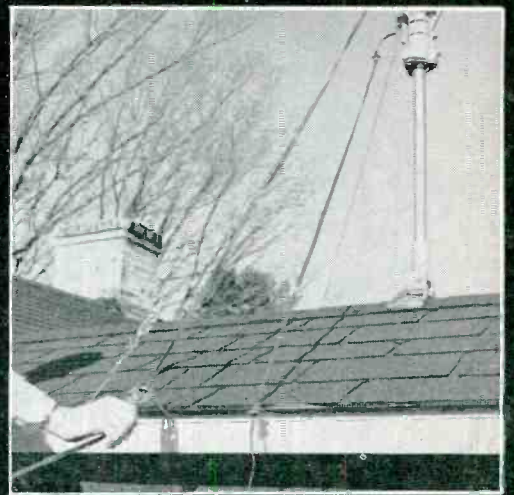
19 Twin-lead and rotator wires should be in standoffs at least 6 inches apart.
