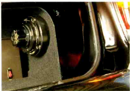
This hefty knob switches system power from the car's battery to the Astron power supplies in the trunk.
