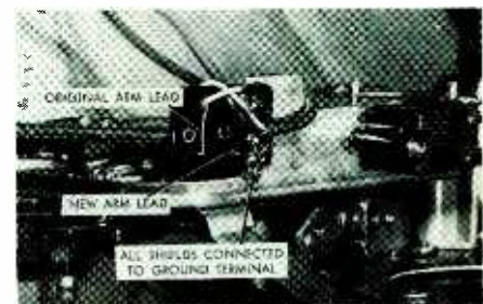
Fig. 2. Shields of two external cables and two arm leads are all connected to the grounding lug. "Hot" leads of external cables are connected on the other side of the switch.
