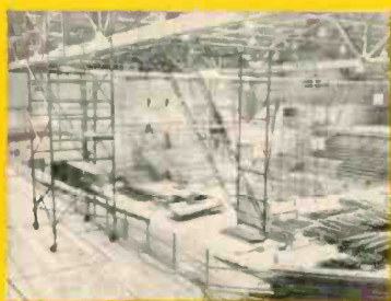
Electro-Voice CDP Public Address Loud-speaker System was chosen for the 8,248 seat North Side Gym, Elkhart, Indiana, one of the nation's largest high school gyms. Cluster of stacked CDP's can be seen in photo taken during construction.
