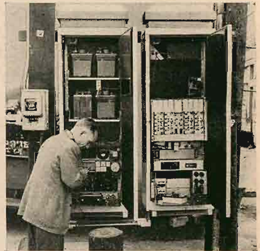
Repeater equipment is mounted at base of pole in cabinet at right, in easy-to-service position. Left-hand cabinet houses emergency power supply. System employs twin-channel technique, transmitting two channels on a single carrier by using upper and lower sidebands. A single oscillator serves two channels.
