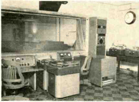
Fig. 2. Control room equipment as seen from student observers' seats. Director's position is at right of turntables, with recording rack and disc recorders at far right. Power supplies, patch panel, and radio tuners are in rack to left of the console.
