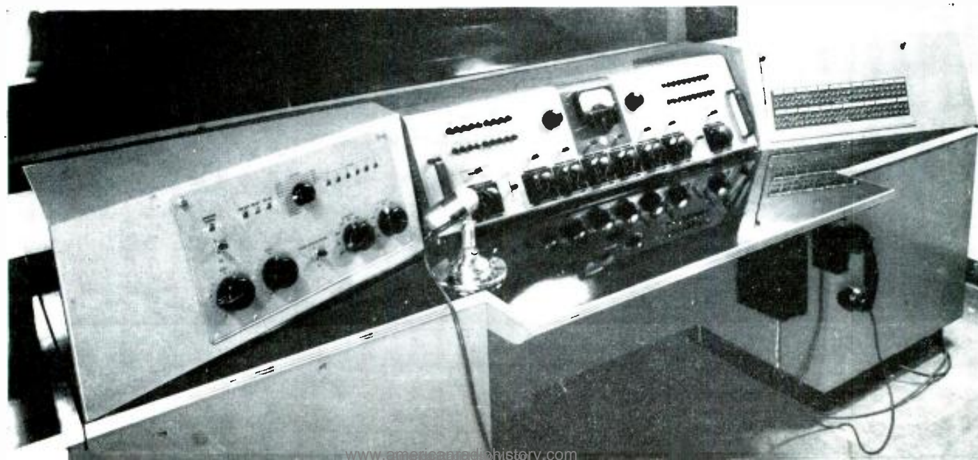
Fig. 5. In Studios C and D, a standard RCA 76-C consolette is used in conjunction with auxiliary custom-built side turrets (jack bay at right—and sound effect filters, echo controls, cue selector and supervisory lights at left). Space is provided for turntables at each side of the operator's position.
