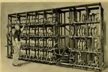
Bank of Ward Leonard Vitrohm plates, controlling the reactore dimmers shown below. The center picture on the opposite page shows this pilot dimmer with the pilot switches and steel front added. This is the largest and finest auditorium in the United States, having a seating capacity of 11,000 persons. The dimmer is the largest in the world. Total load connected to dimmers, 900 kw. The pilot board shown in the center of the opposite page controls the contactor board in the basement. This was built by the Cleveland Switchboard Company.
