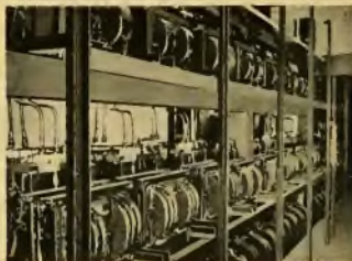
The Ward Leonard Reactore Dimmers installed at the rear of the contactor board in the basement of the Cleveland Auditorium. These are controlled by the bank of Vitrohm plates, shown above, and regulate the lamps of stage and house from full brilliancy to maximum. This is the first installation of its kind and has been in operation for about nine years giving perfect satisfaction.
