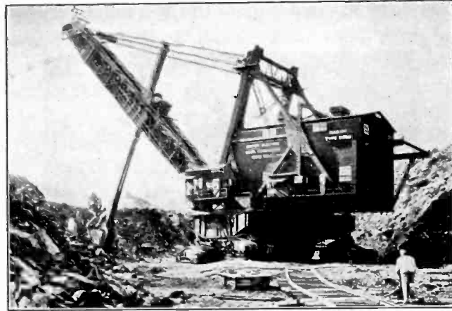
FIG. 13—THIS ELECTRIC SHOVEL HAS A SCOOP CAPACITY OF 15 TO 20 CU. YD. AND WEIGHS 1800 TON
