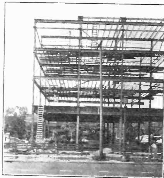
FIG. 1—CLEVELAND OFFICE BUILDING. ILLUSTRATES DECREASE IN WEIGHT OF COLUMNS FROM THE FIRST FLOOR TO THE FOURTH FLOOR
