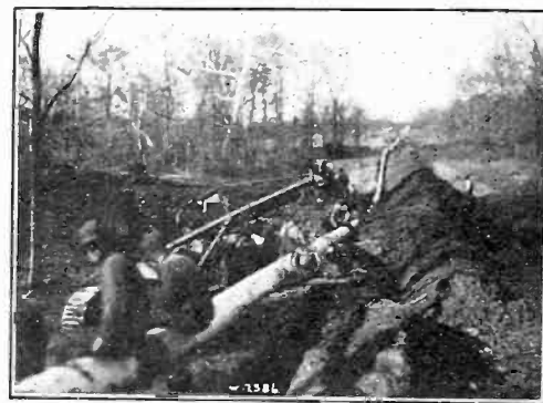
FIG. 6—BELL HOLE WELDING ON 12-IN. PIPE LINE NEAR WELCH, OKLAHOMA. OBSERVE BENDS IN PIPE DUE TO UNEVEN TERRAIN, WHICH CAUSES NO FAILURES
