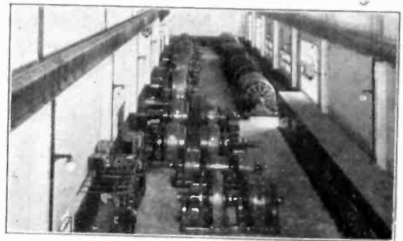
FIG. 4—GENERAL VIEW OF THE MOTOR ROOM AT THE 14-IN. MERCHANT MILL OF THE JONES AND LAUGHLIN STEEL CORPORATION, WOODLAWN, PA.
