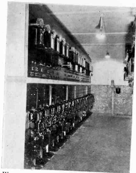
FIG. 10—WOODHAVEN SUBSTATION 4000-VOLT OIL CIRCUIT BREAKERS AND CONTROL PANELS
