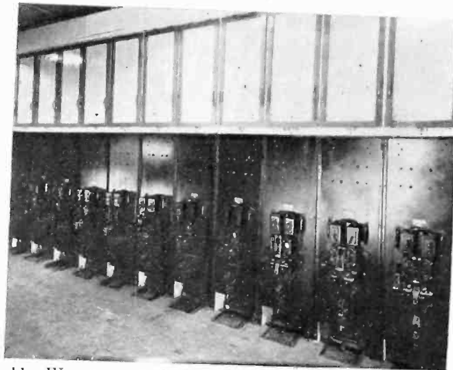
FIG. 11—WOODHAVEN SUBSTATION, 13,200-VOLT OIL CIRCUIT BREAKERS
