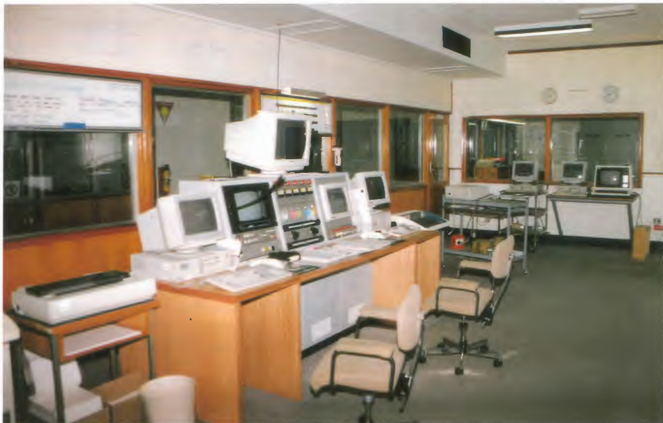
New control desk. Original Ramtek monitors have been replaced by PC's. Computer terminals for three Collins 250kW transmitters at end of room.
