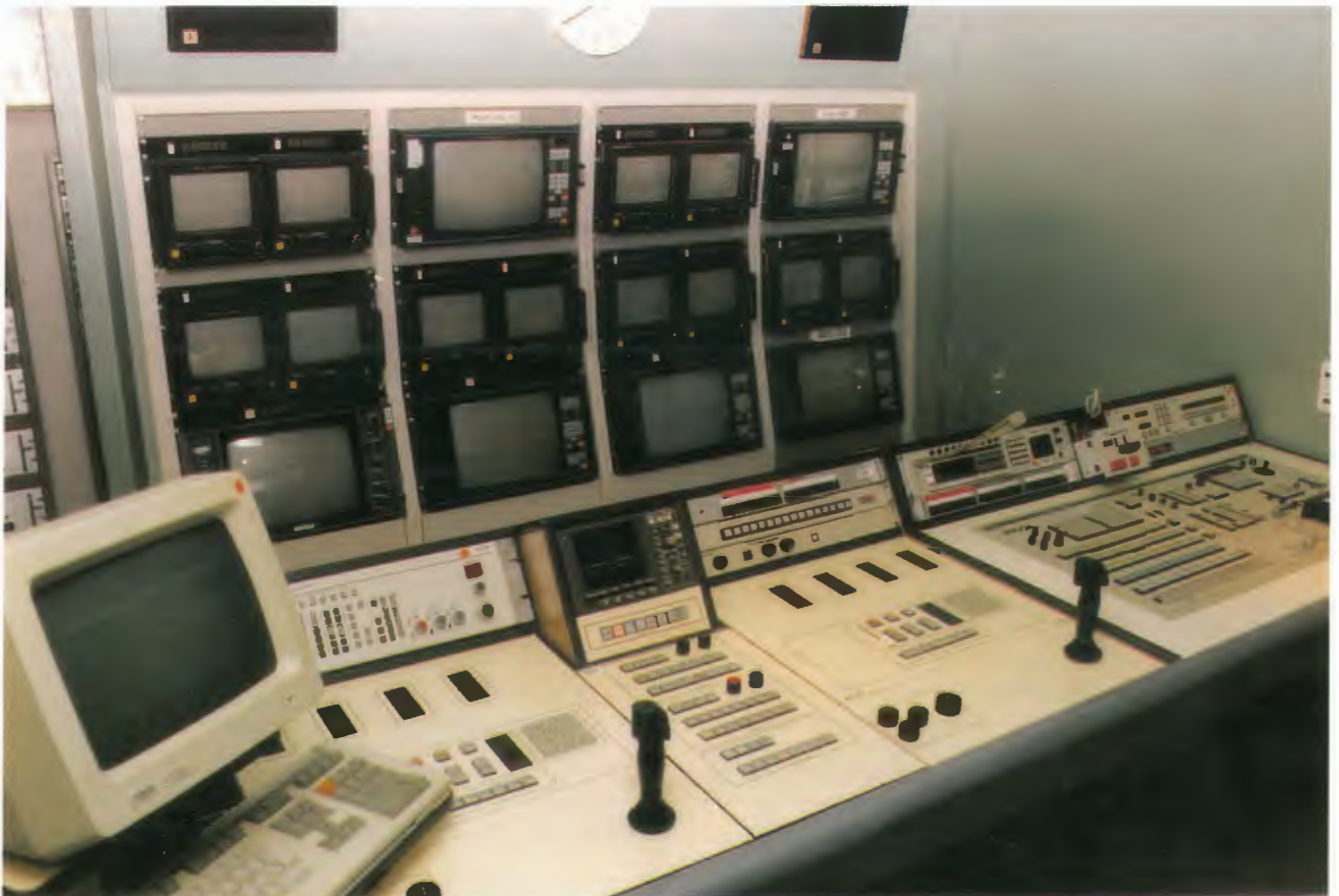
HOUSE of REPRESENTATIVES, Vision Control Room (Vinten Remote Camera Pan and Tilt Head Joysticks in Foreground)
