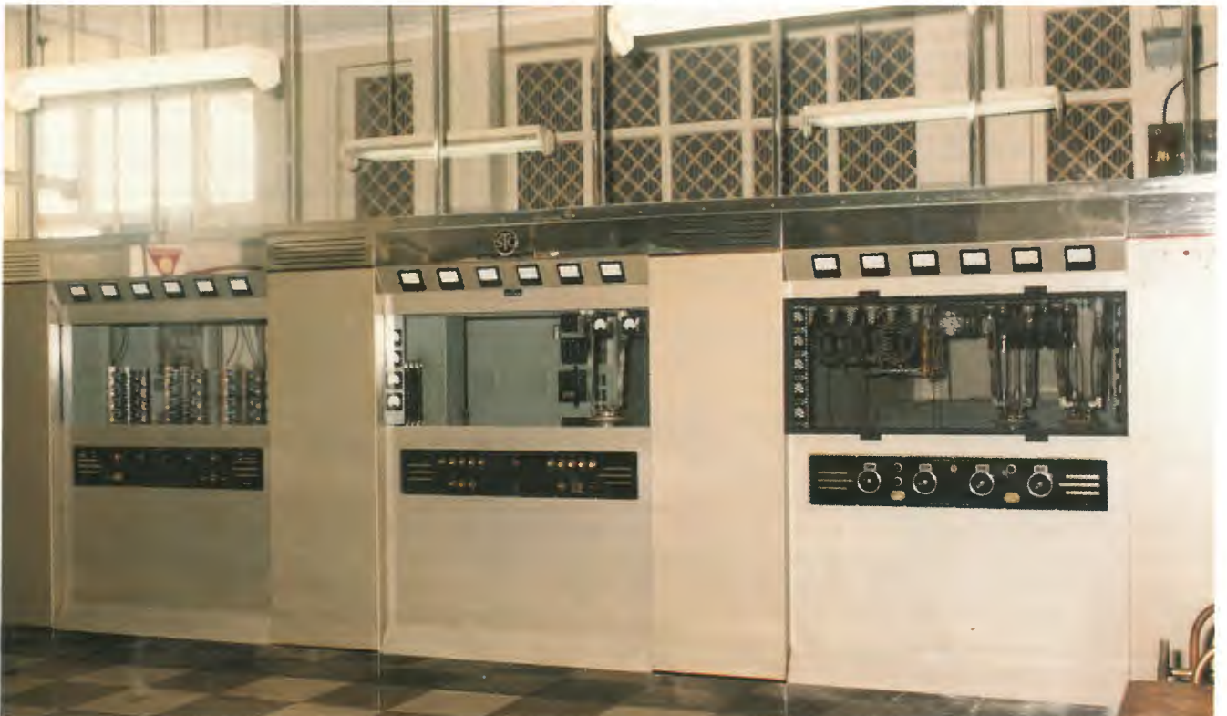
Present 2NR 50 kW transmitter.
