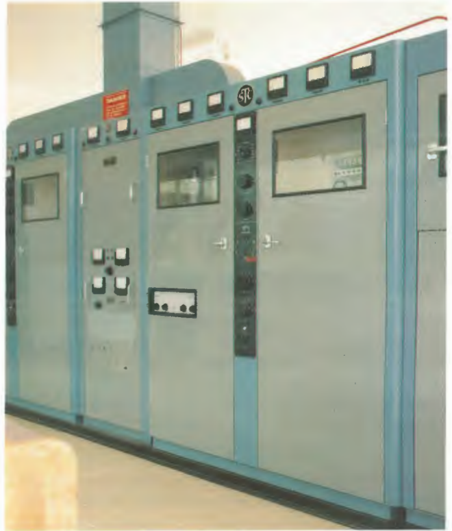
The replaced STC 2x5 kW transmitter.
