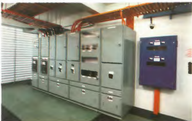
Main power board and battery chargers.
