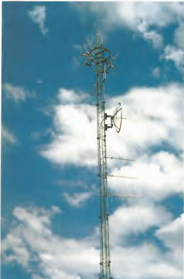
The station mast and aerial systems.
