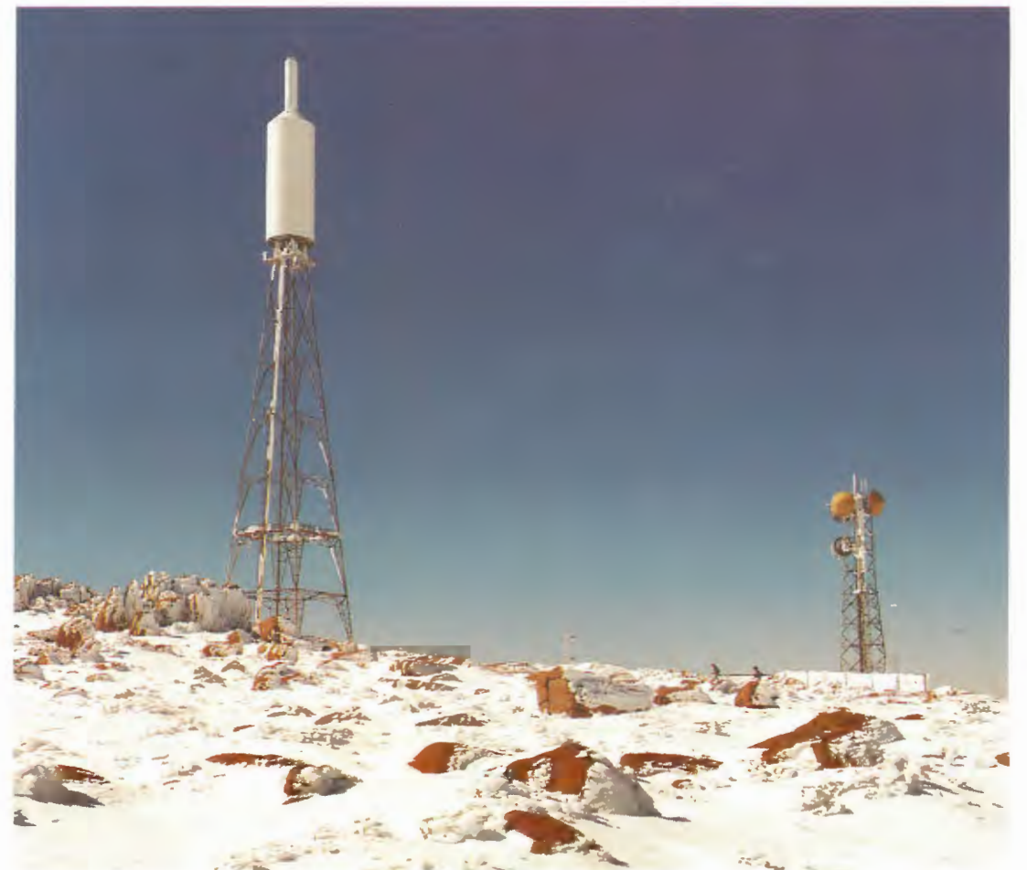
National transmitter site and Telecom R/T site on right.
