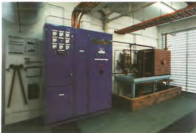
Emergency supply power board and day service tank.
